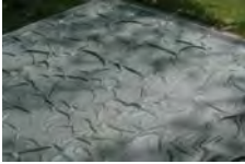
Poorly Adhered Membrane
