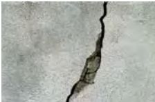
Cracks in Concrete
